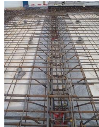
Figure 4: An example of a thickened slab. The “thickening” is actually a cast-in-place footing to support line loads directly above.
