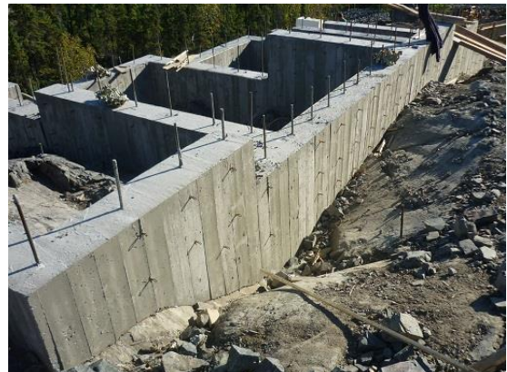
Figure 3: This stepped footing actually is the foundation wall as well, because the bedrock is competent, so a spread footing is not needed to transfer loads.
